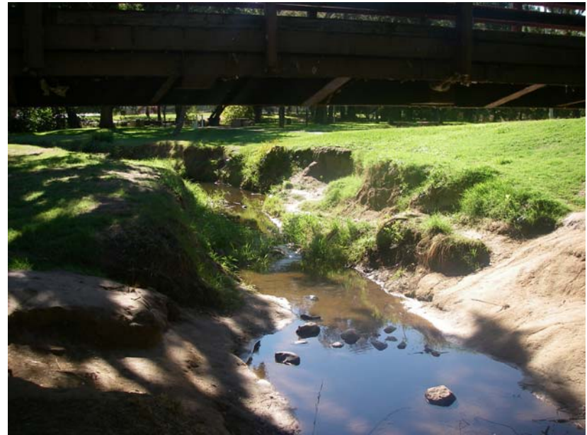
Eroding Bank near Bridge in Rusch Regional Park (Reach 26)
