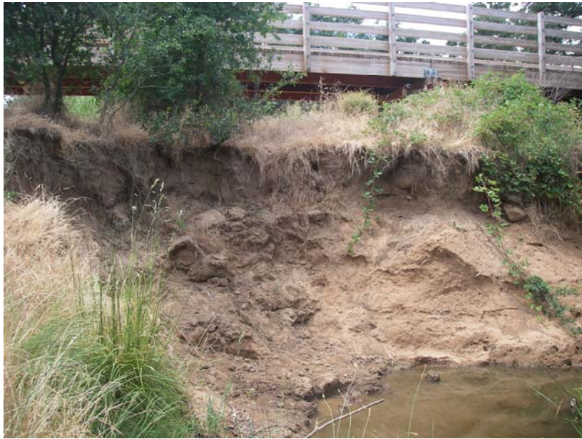
Severe Bank Erosion on Left Bank Adjacent to Pedestrian Bridge (Reach 16)
