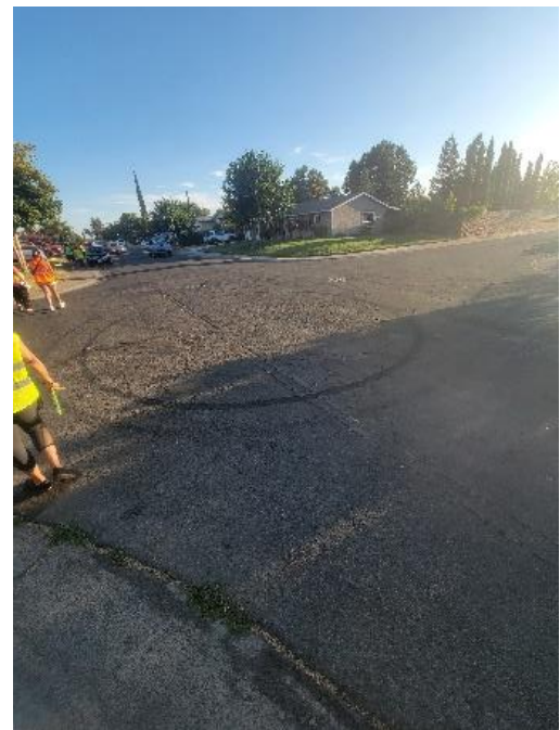
Figure 40. Tire Marks at 68th Avenue and Balfour Way
