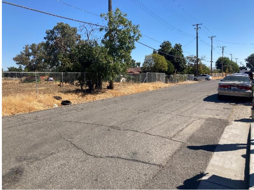
Figure 30. Missing Sidewalk along 63rd Street
