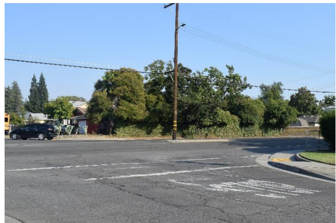
Figure 24. Faded Crosswalk at 18th Avenue and 65th Street Expressway.
