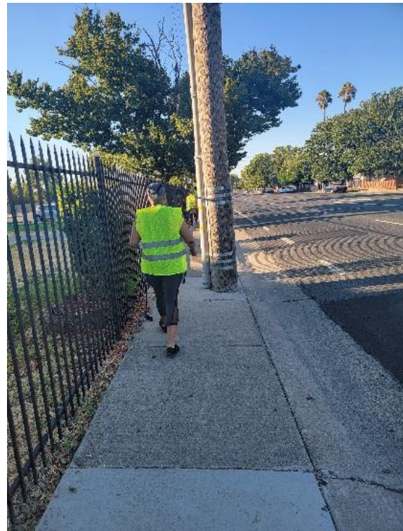
Figure 38. Utility Pole Obstructing the Pedestrian Right-Of-Way along 24th Street
