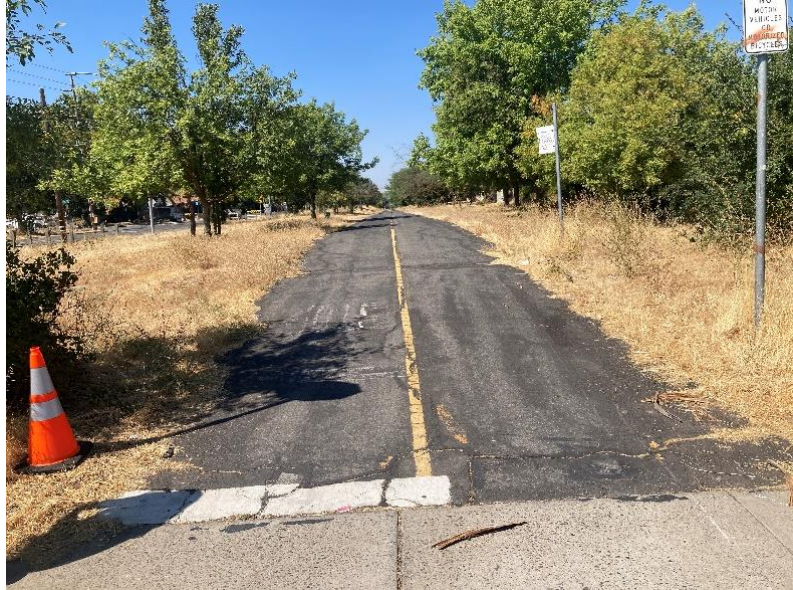
Figure 9. Maintenance Issues along North Sacramento Bike Trail
