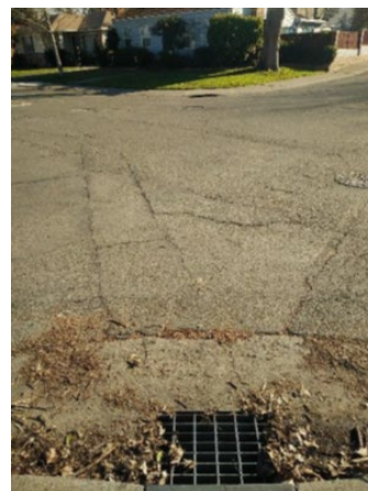
FIGURE 12. DEBRIS COLLECTING ON A STORM DRAIN AT THE CORNER OF 45TH AND C STREETS
