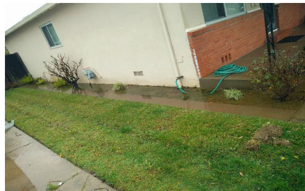
FIGURE 31. PONDING CAUSED BY LANDSCAPING OBSTRUCTIONS
