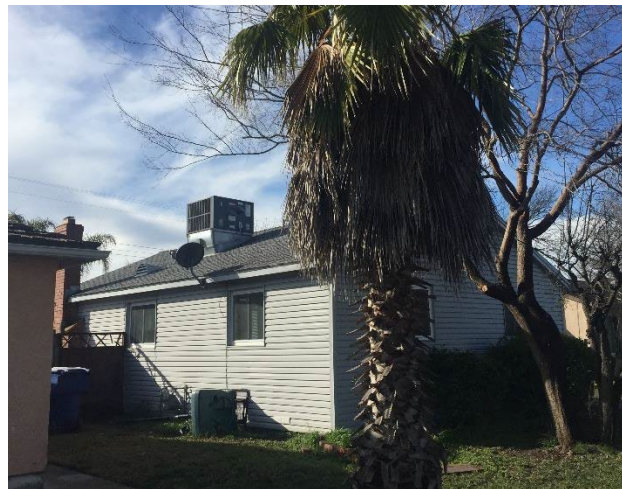
FIGURE 41. EXAMPLE OF UTILITIES LOCATED ON THE ROOF; MANY OF THE HOMES IN THIS AREA HAVE HVAC UNIT LOCATED ON THE ROOF
