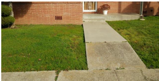
FIGURE 36. CRAWL SPACE UTILIZED AS A FLOODPROOFING MEASURE TO PREVENT FLOODING IN THE STRUCTURE
