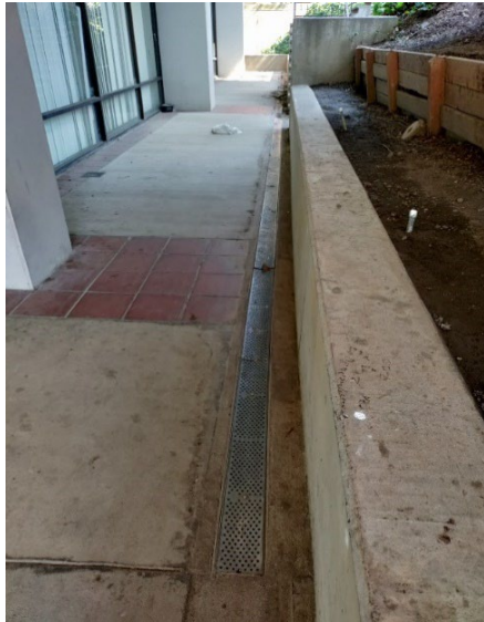
FIGURE 27. TRENCH DRAINS ALONG SOUTH SIDE OF LOWEST FLOOR
