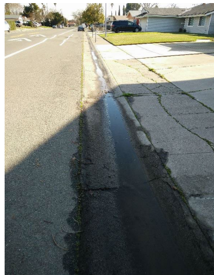
FIGURE 37. STANDING WATER AFTER A LARGE JANUARY STORM UNABLE TO CONVEY FLOWS
