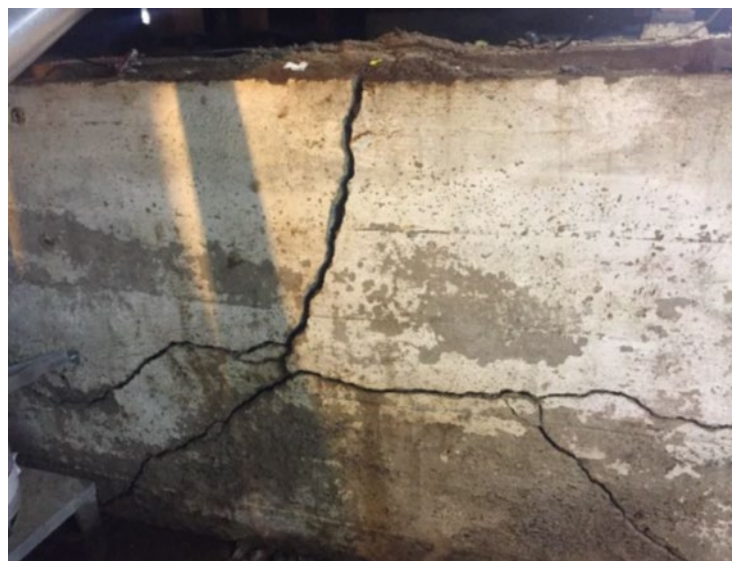
FIGURE 18. A FRACTURED BASEMENT WALL CAUSED BY HYDROSTATIC PRESSURE; CRACKS HAVE LED TO WATER SEEPING INTO THE BASEMENT
