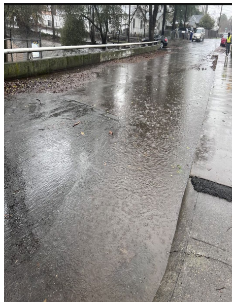
FIGURE 48. VERANO BRIDGE WATER PONDING
