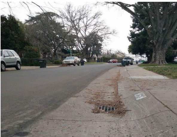
FIGURE 19. EXAMPLE OF DEBRIS IN THE STORM DRAIN. LEAF PILES ARE ALLOWED TO BE LEFT ON STREETS FOR CITY PICKUP AFTER CURBSIDE BINS ARE FULL; MANY TIMES, THESE LEAVES CAN CLOG THE STORM DRAIN
