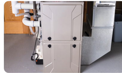
Gas Furnace: 80,000 Btu single-stage gas furnace
