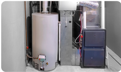
Gas Water Heater: 40-gallon storage tank
