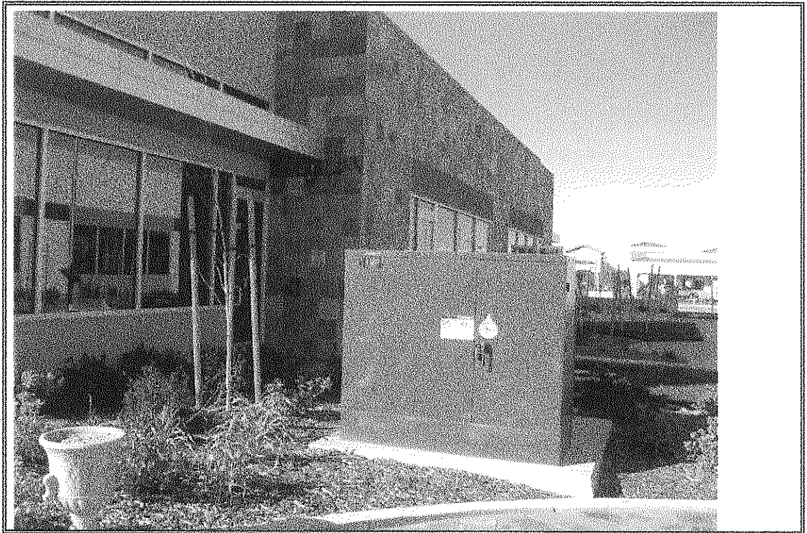
Photograph Number 14 Transformer east of 2250 Building
