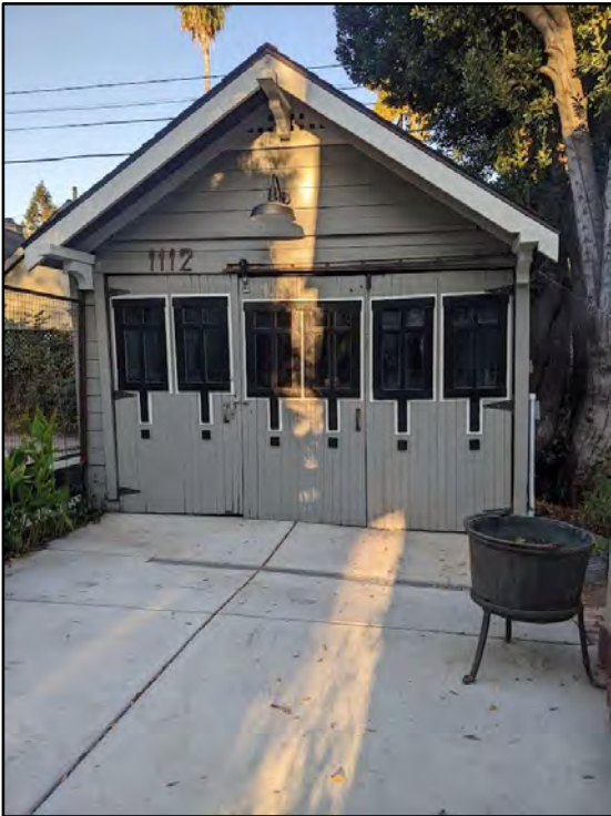
The original garage has an unusual quantity of Craftsman detail on its façade, East Elevation.
